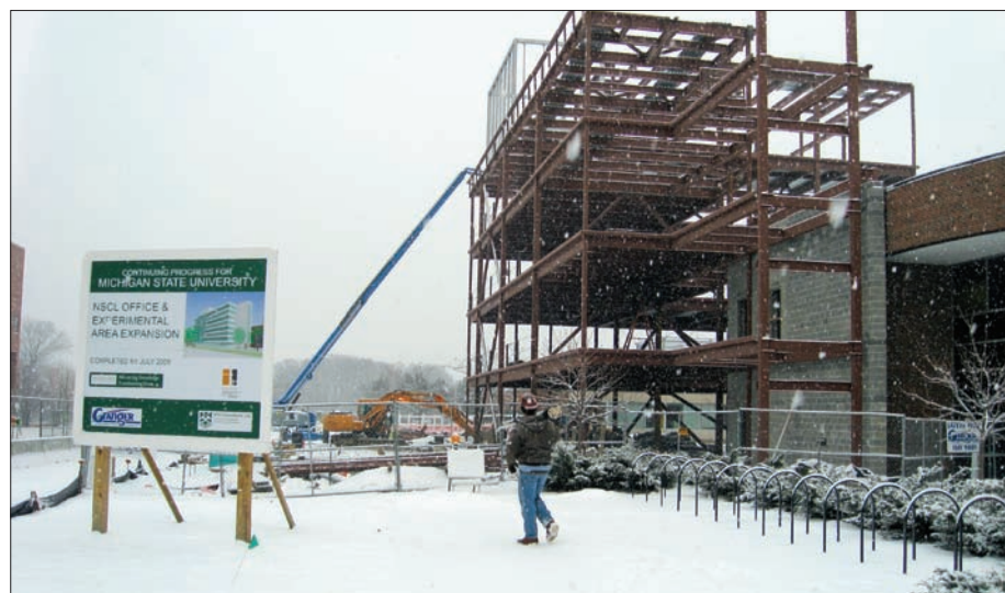
Work on the steel structure of the new offices at NSCL started on 15 December 2008. (Courtesy NSCL.)
